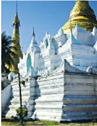
Over 60 terracotta jataka plaques, featuring the last ten tales, were once placed inside niches on the terrace. The base and terraces were plastered and whitewashed in the early 20th century. Only some ten plaques survive in situ.
