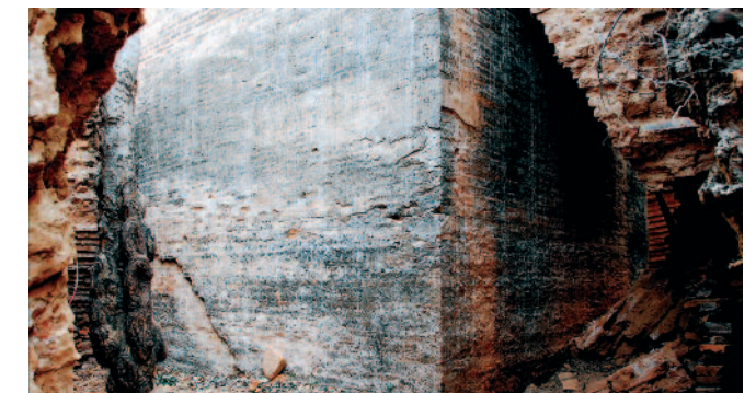
This solid brick blockhouse once capped the pagoda. The centre of the flat roof collapsed inward at the time of the 1838 earthquake, causing the blockhouse to plunge inside the pagoda. It was originally supported by four corbelled arches that were concealed immediately below the roof. These arches prove that the blockhouse was part of the original design and perhaps suggests that the builders had completed the pagoda.
