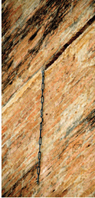
The plaster which concealed the horizontal rows of chains has come out in some spots and bits of chain dangle down the walls of the structure.
