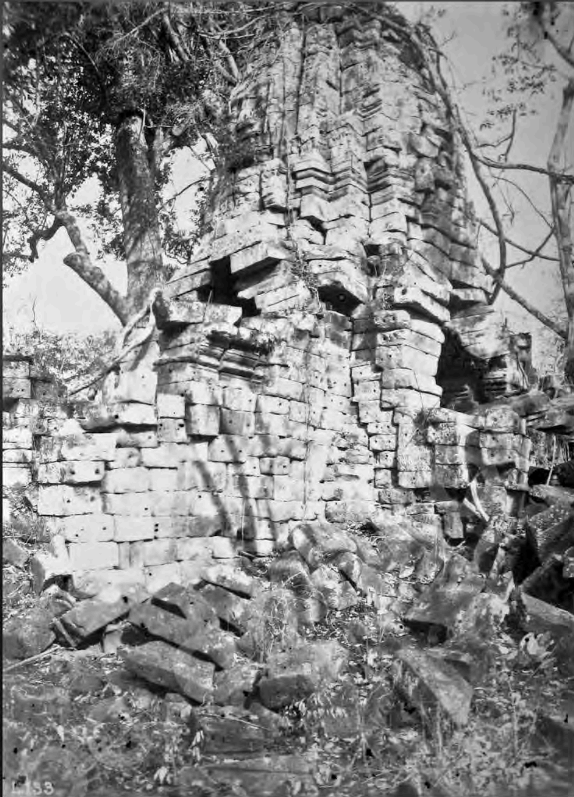
Condition of the South and East side of the face tower of the satellite-temple VII in February 1932 (G. Groslier - © MCFA - 129.13)
