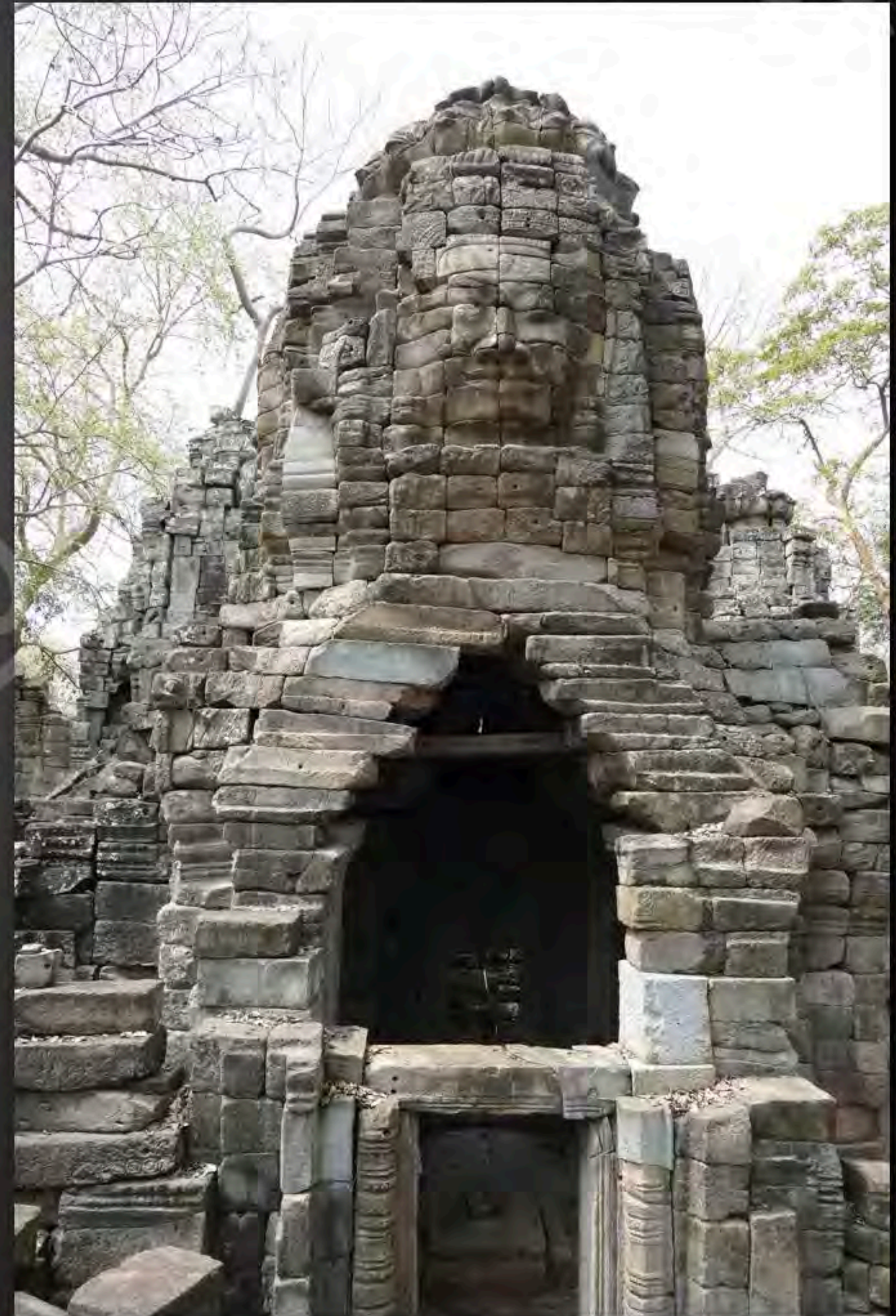
Current condition of the East side of tower 18 of the 1 st enclosure after restoration by the GHF between 2010 and 2014 (February 2015)
