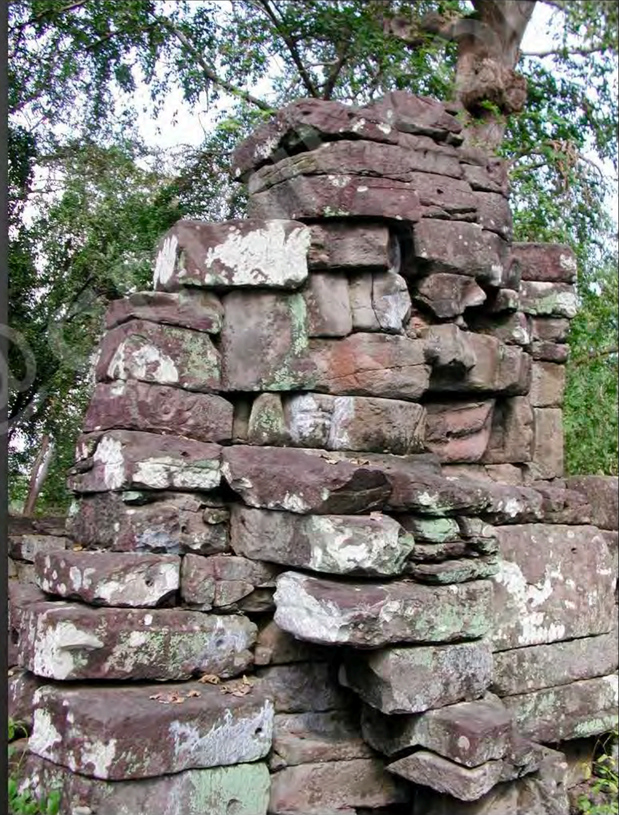
Current condition of the South side of tower 20 of the 1 st enclosure (December 2002)
