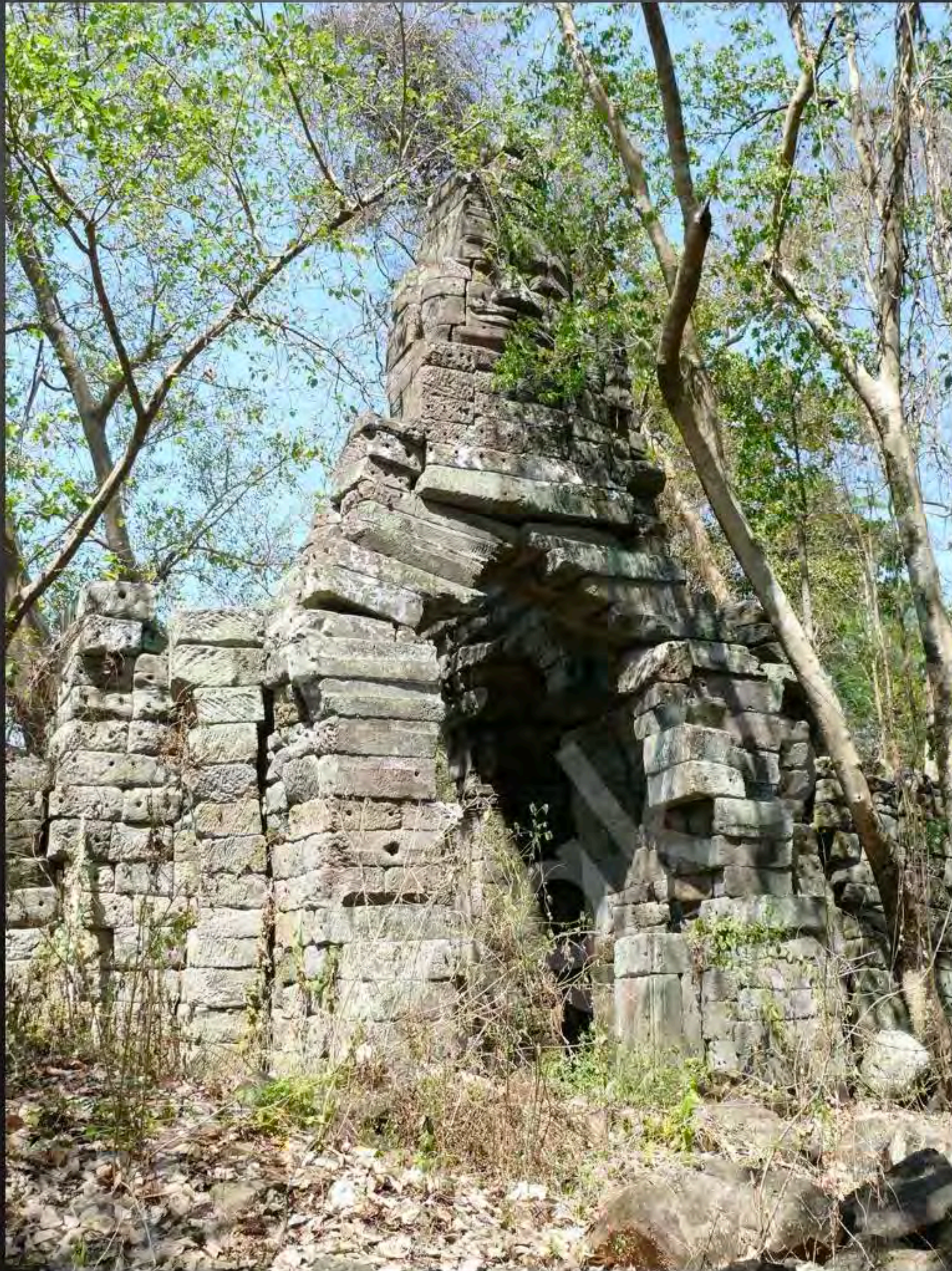
Current condition of the East side of the face tower of the satellite-temple III (March 2010)
