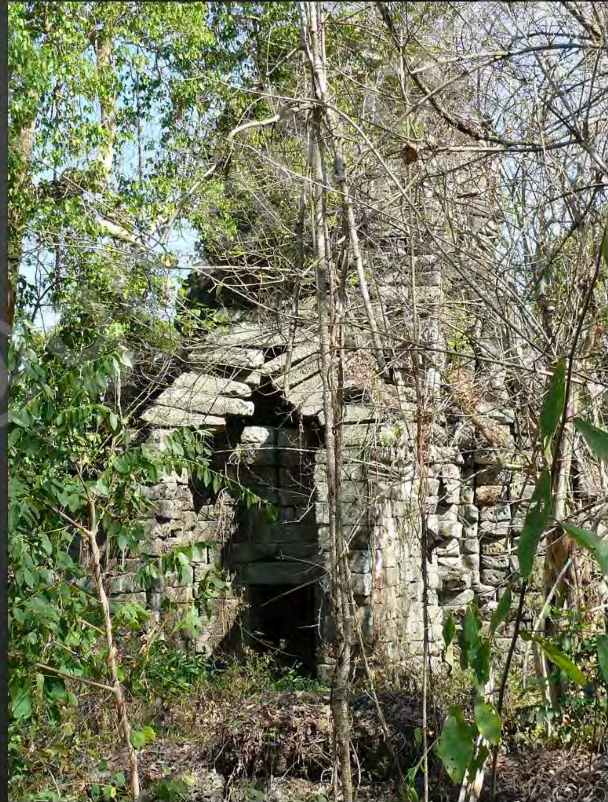
Current condition of the South side of the face tower of the satellite-temple V (March 2010)
