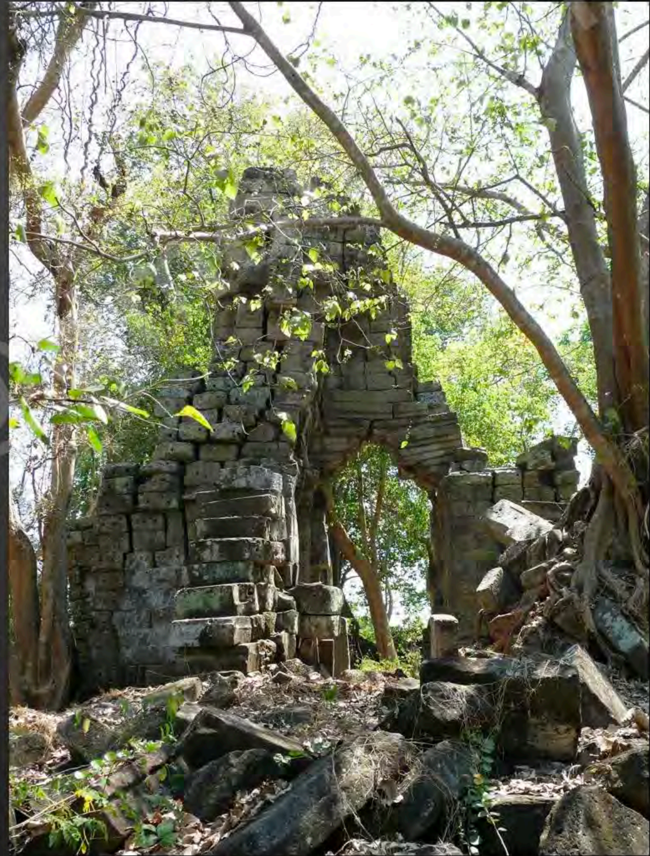
Current condition of the West side of the face tower of the satellite-temple III (March 2010)
