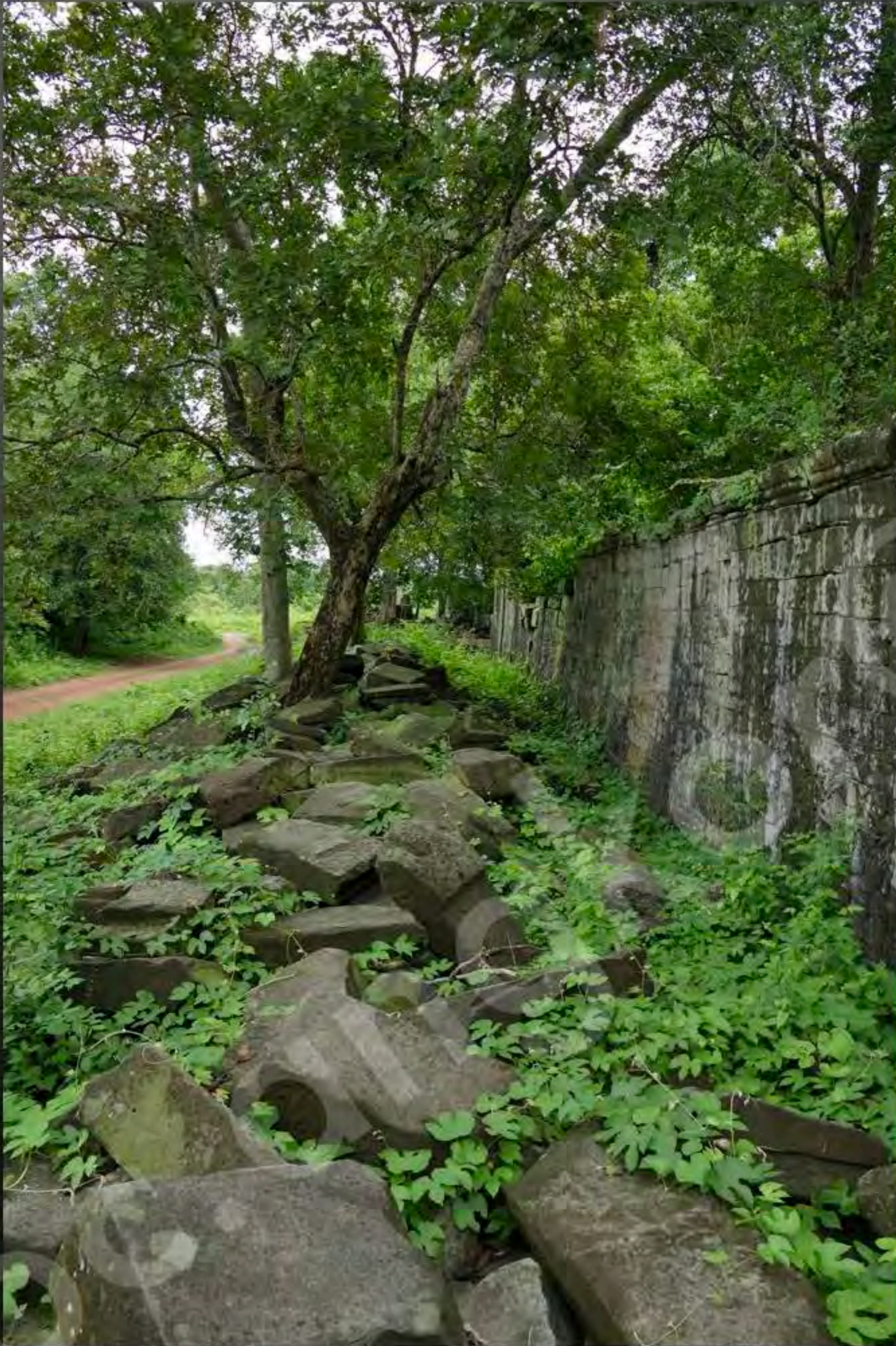
Current condition of the East wing of the Northern gallery View from West to East (September 2015)
