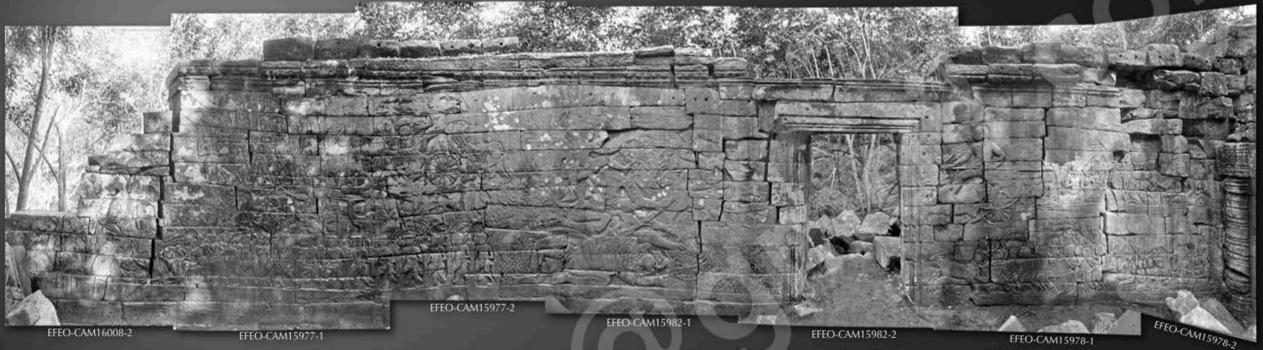
Condition in 1909 of the South end of the North wing of the Western gallery (Photomontage of the photos of General de Beylié from the photos archives of the EFEO)
