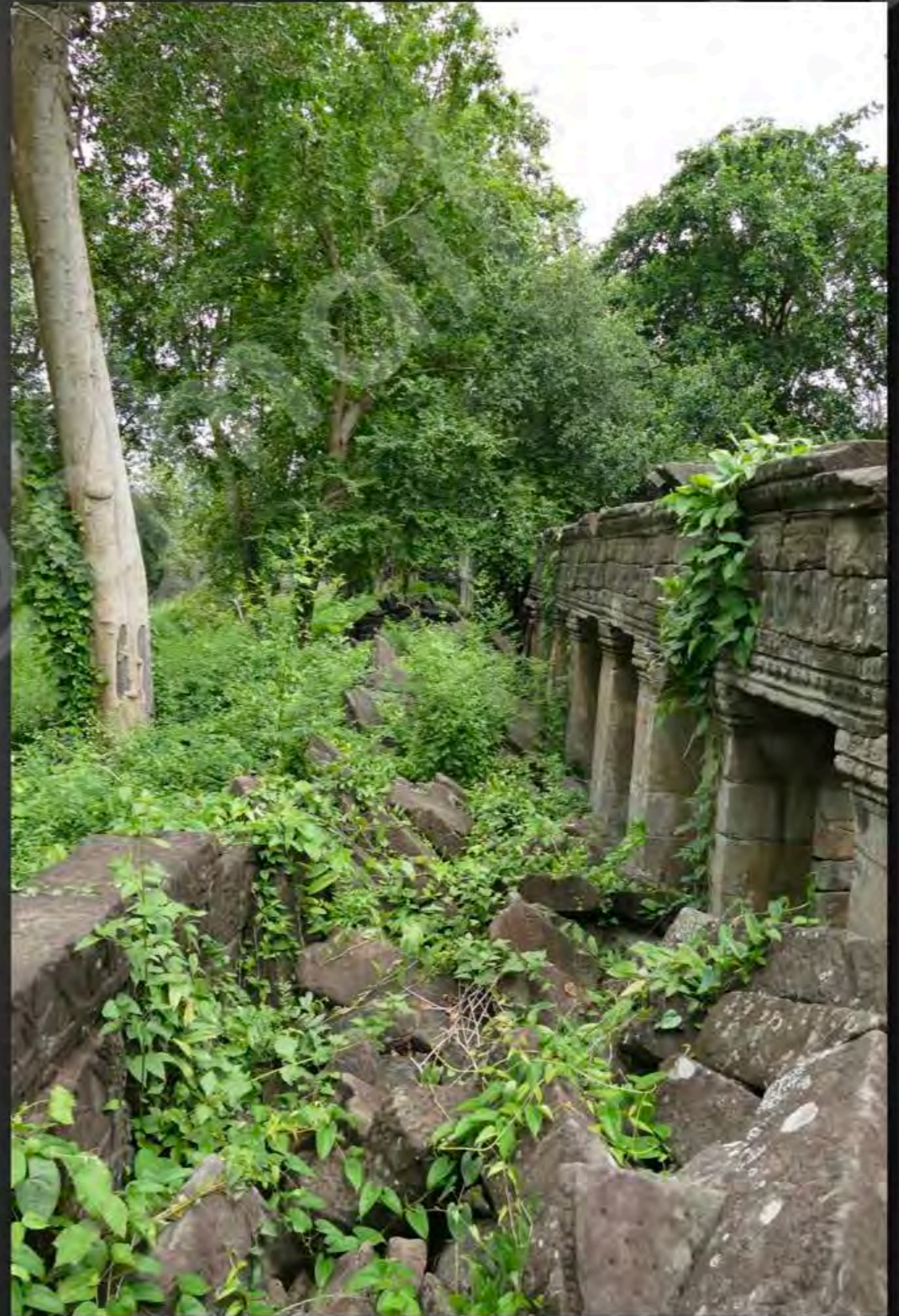
Current condition of the East wing of the Southern gallery View from West to East (September 2015)
