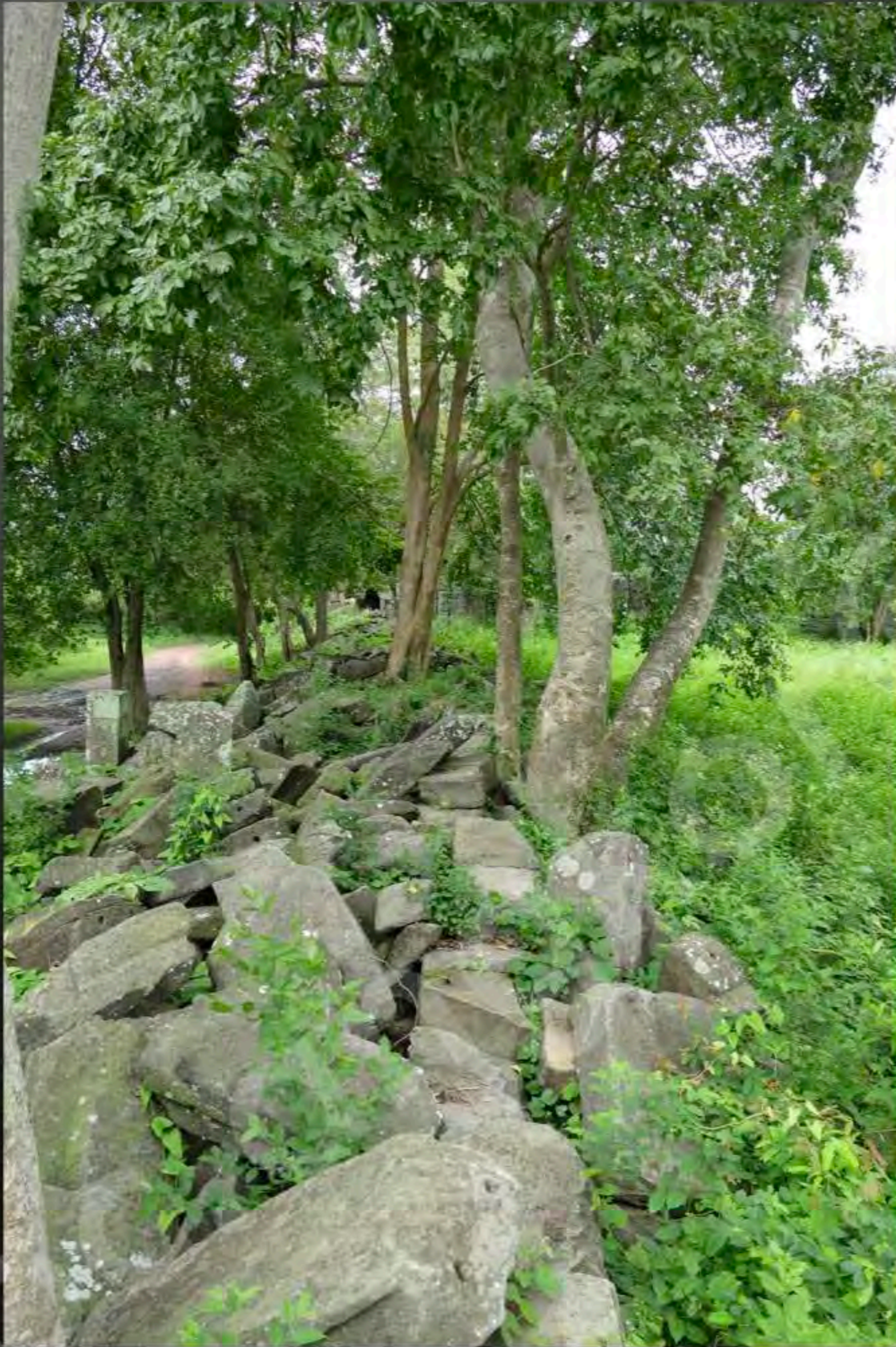
Current condition of the West wing of the Southern gallery View from East to West (September 2015)
