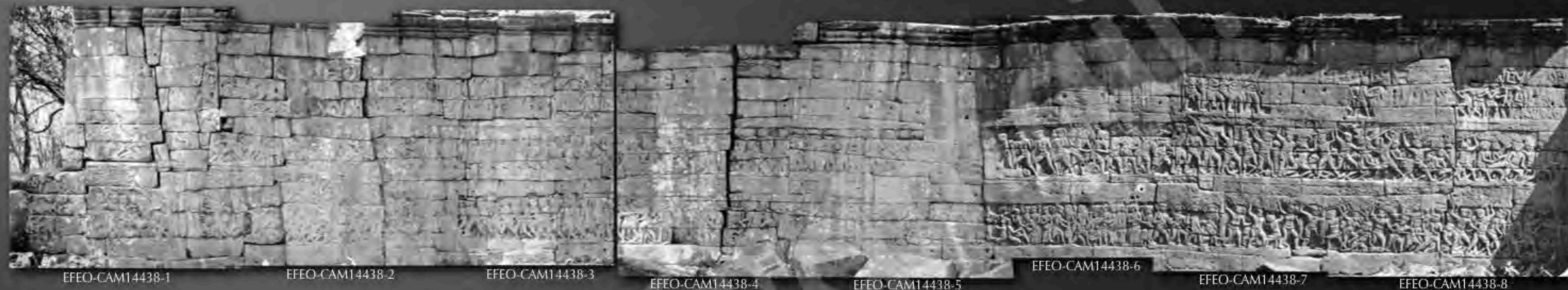
Condition in 1965 of the East part of the West wing of the Southern gallery (Photos of Luc Ionesco from the photos archives of the EFEO)
