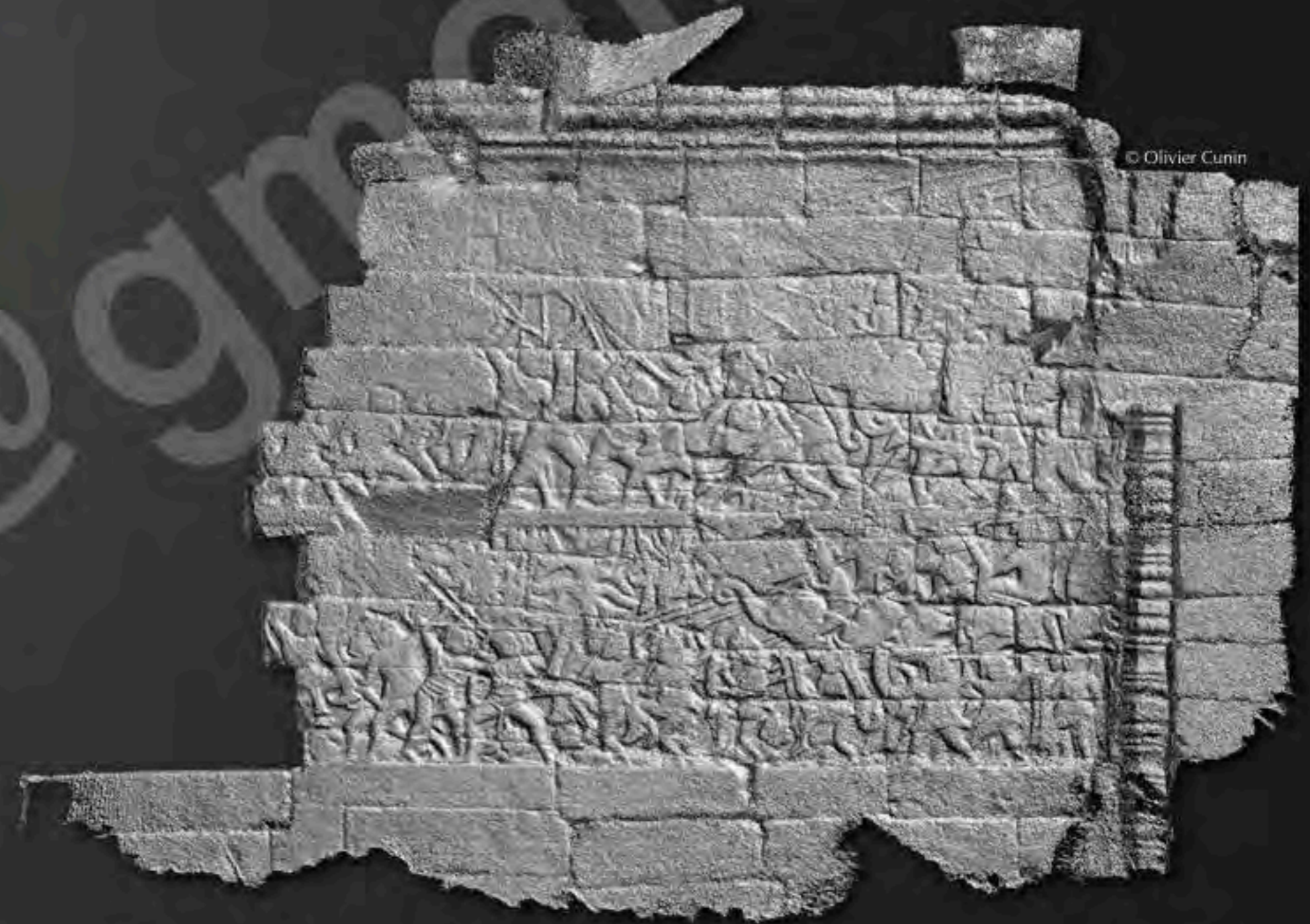
3D scanning by photogrammetry of the current condition of the East end of the East wing of the Southern gallery
