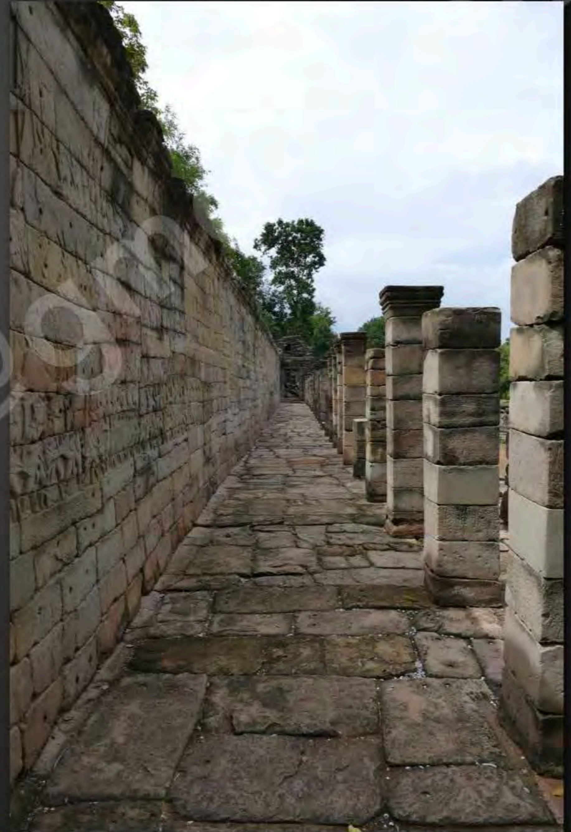
Current condition of the South wing of the Eastern gallery View from South to North (September 2015)
