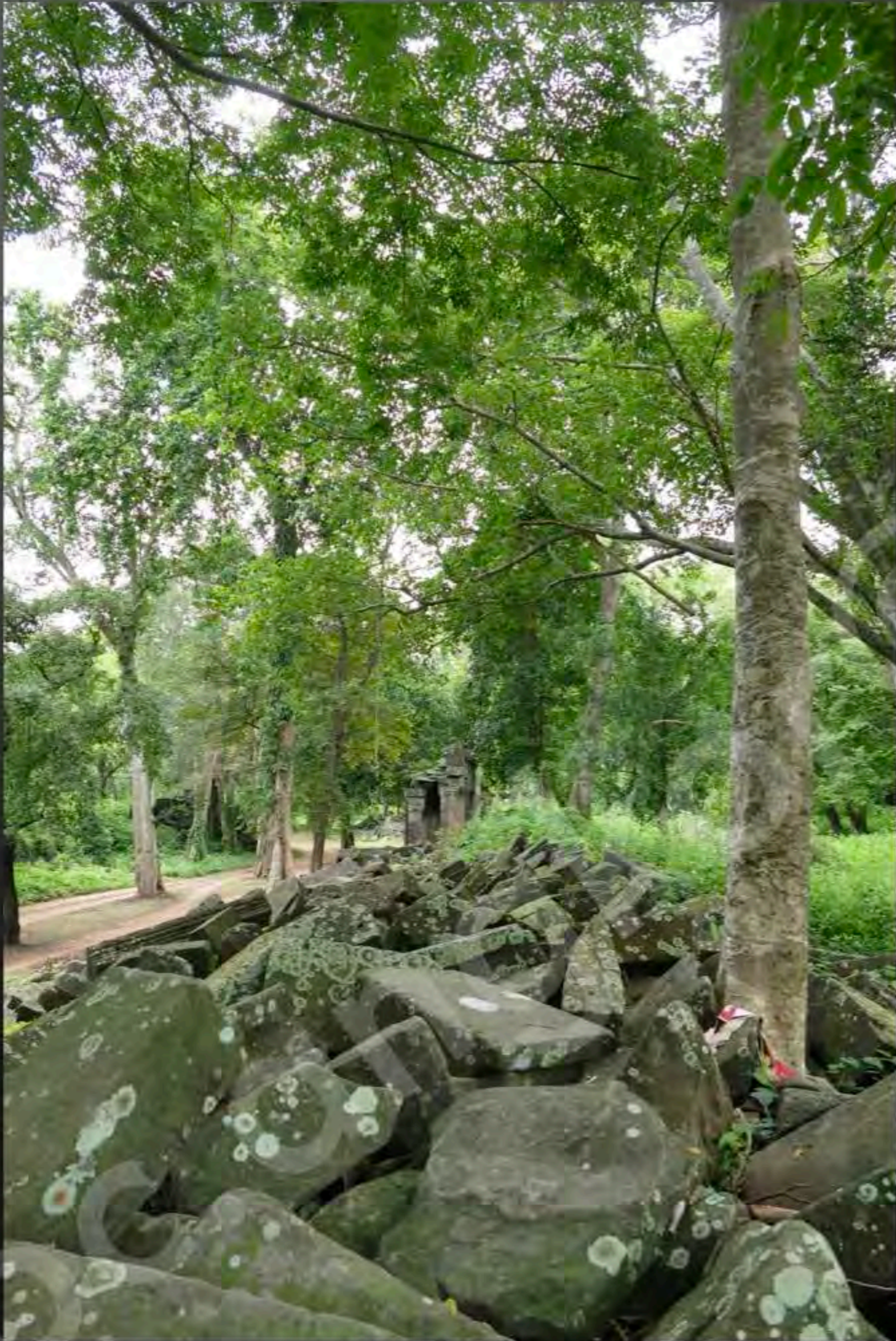
Current condition of the East wing of the Southern gallery View from East to West (September 2015)
