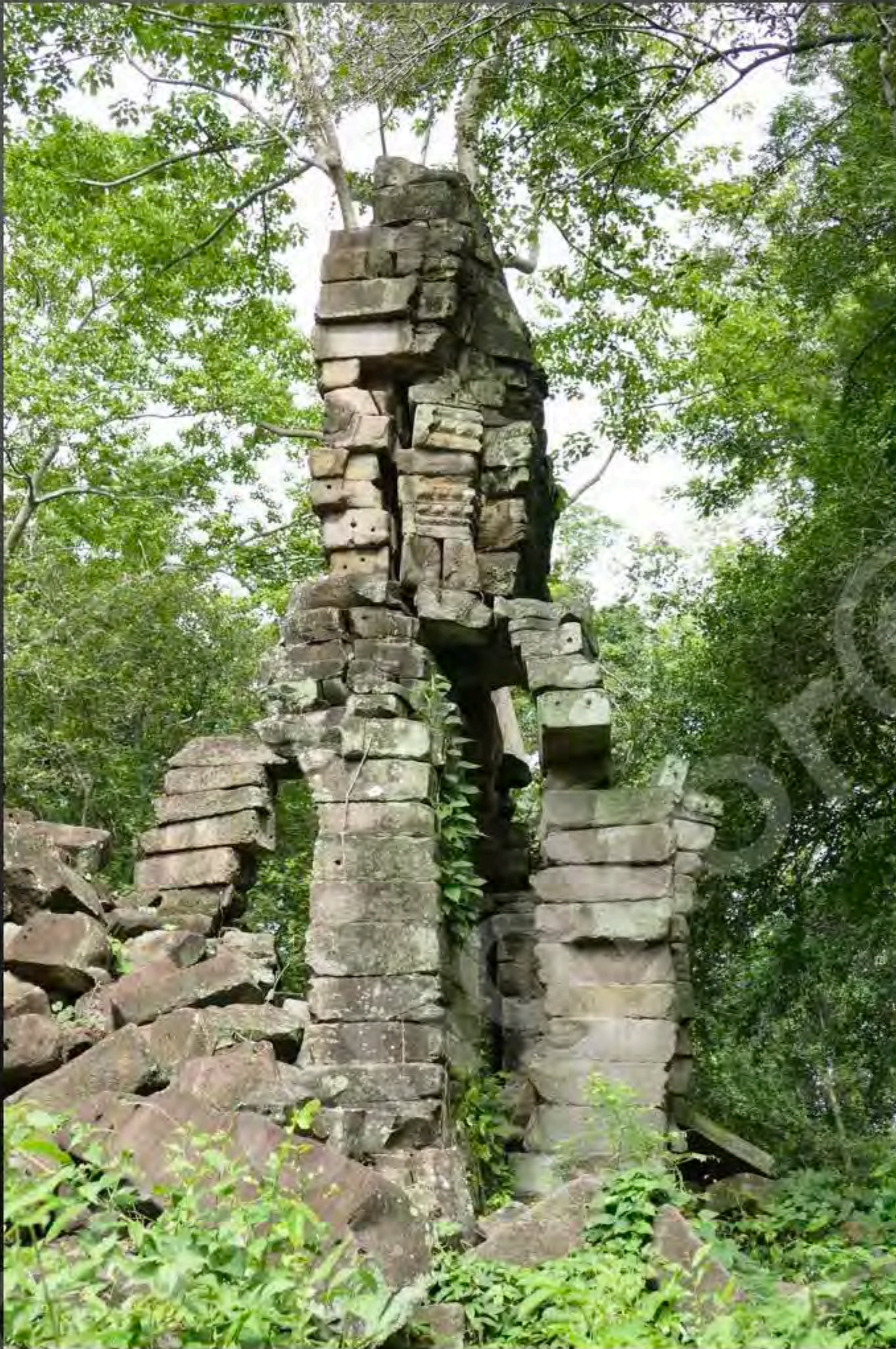
Current condition of the West side of tower 70 of the Western of the 2 nd enclosure (September 2015)
