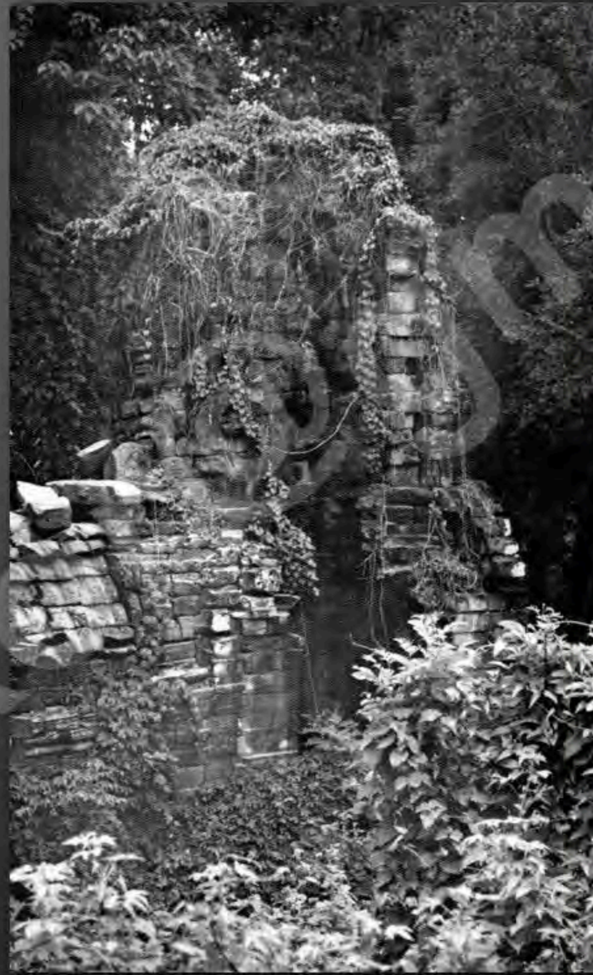
Photo of the tower 70 of the Western of the 2 nd enclosure view from the Northwest in 1992 by Christophe Pottier (CP-SRP-27-26)
