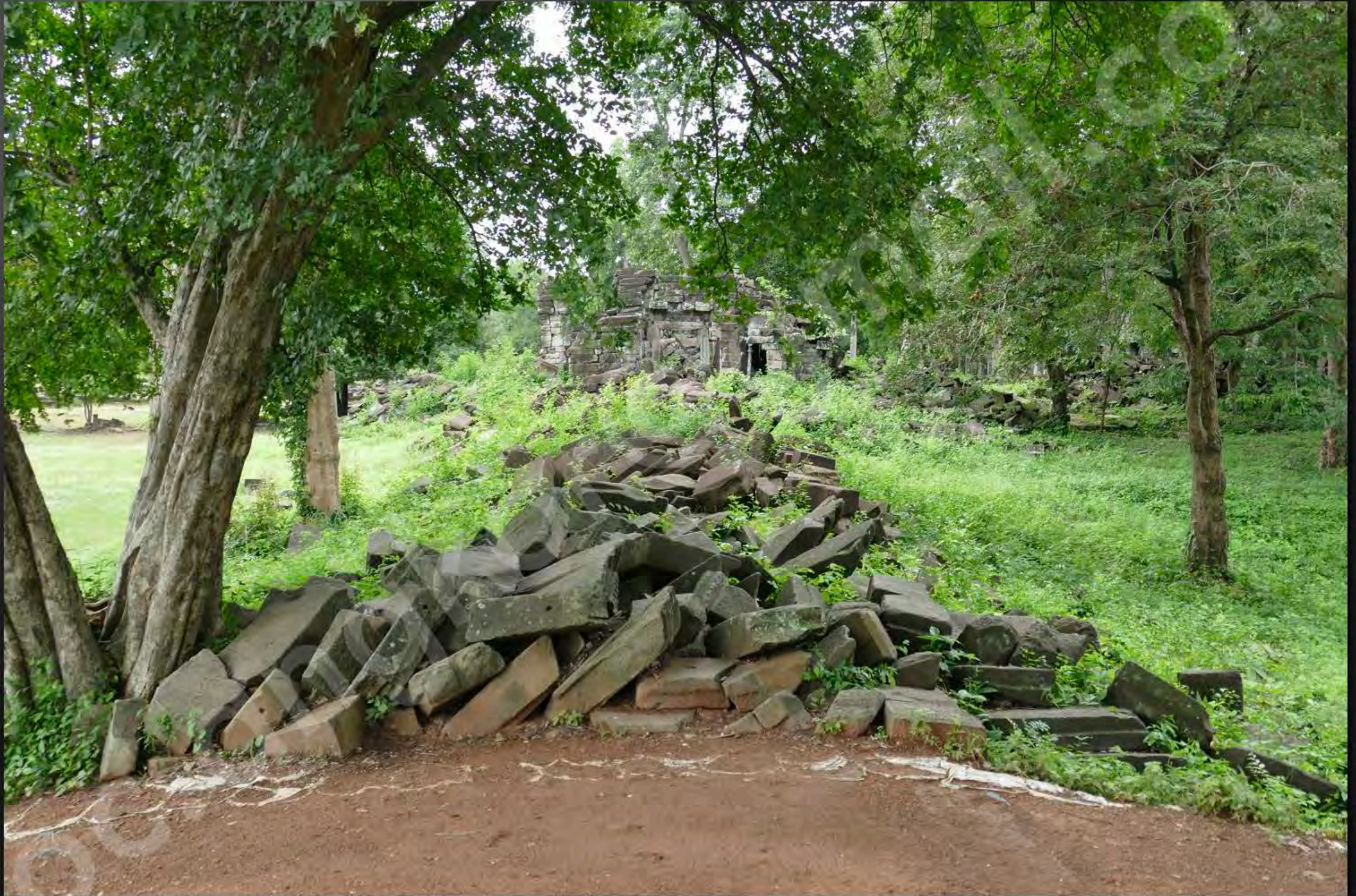
Current condition of the North wing of the Eastern gallery View from North to South (September 2015)
